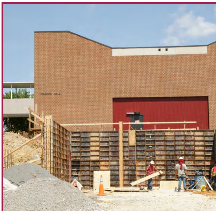
Concrete forms are now in place on the site of phase two of the Snyder Auditorium project.
